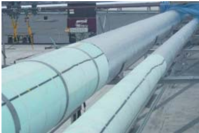
Typical thermally insulated pipe.
