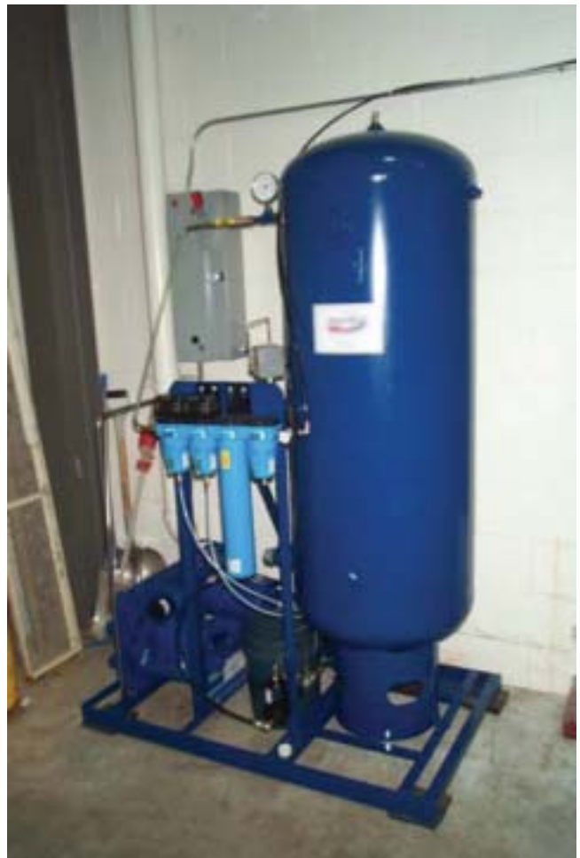
DAI equipment—compressor, filters, and dryer.
