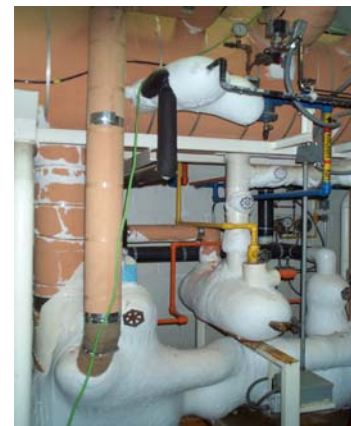
External icing due to water infiltration.
